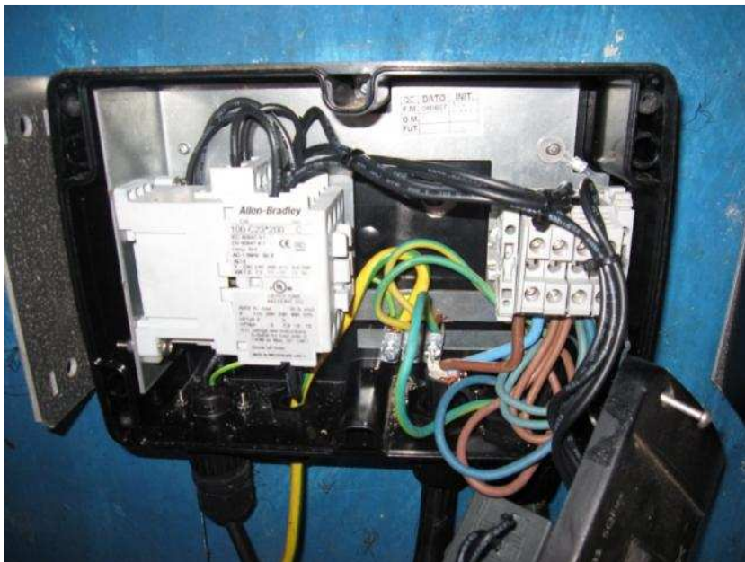
Inside the Grundfos IO101 after the connections were in place. The white box on the left is the relay for automatic switching between solar and generator power.
