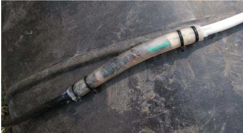
One of the cable joints on the main power cable.
