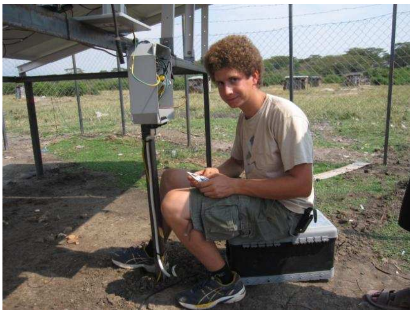
Valentin Koestler having been responsible for the installation of the solar system is doing electrical connections in the control box for the solar panels.
