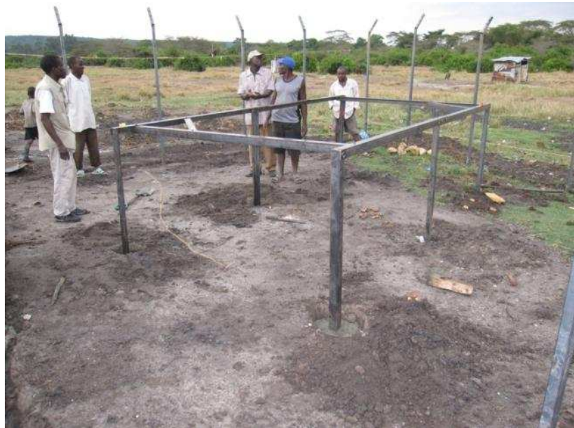
The frame being aligned within the compound and concrete was poured around the legs.
