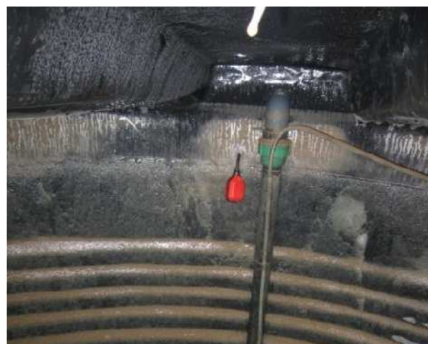
The level switch (red) mounted inside the settlement tank.
