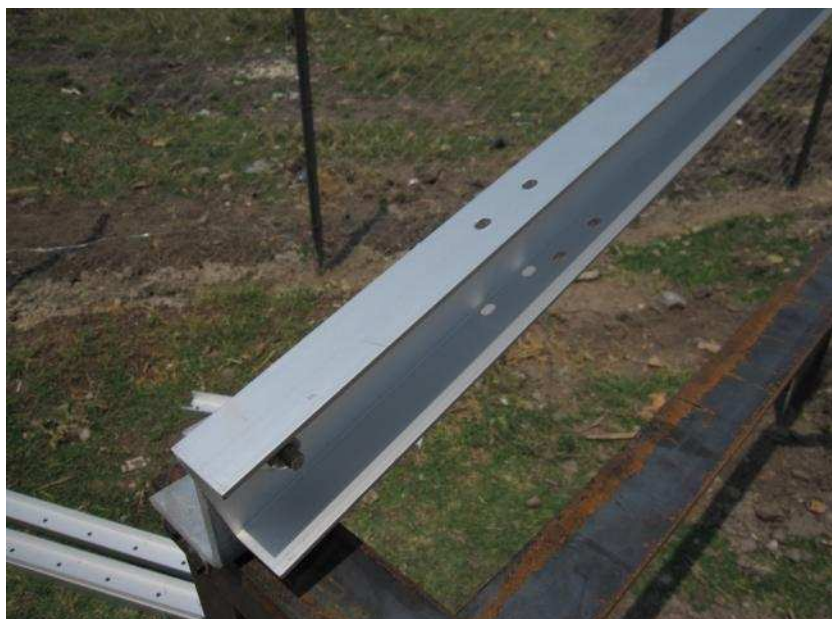
The slightly offset holes in the support girders.
