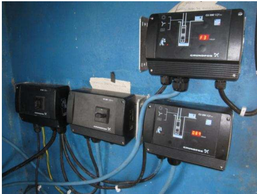
The control boxes while operating. The panels are currently producing 0.89 kW.
