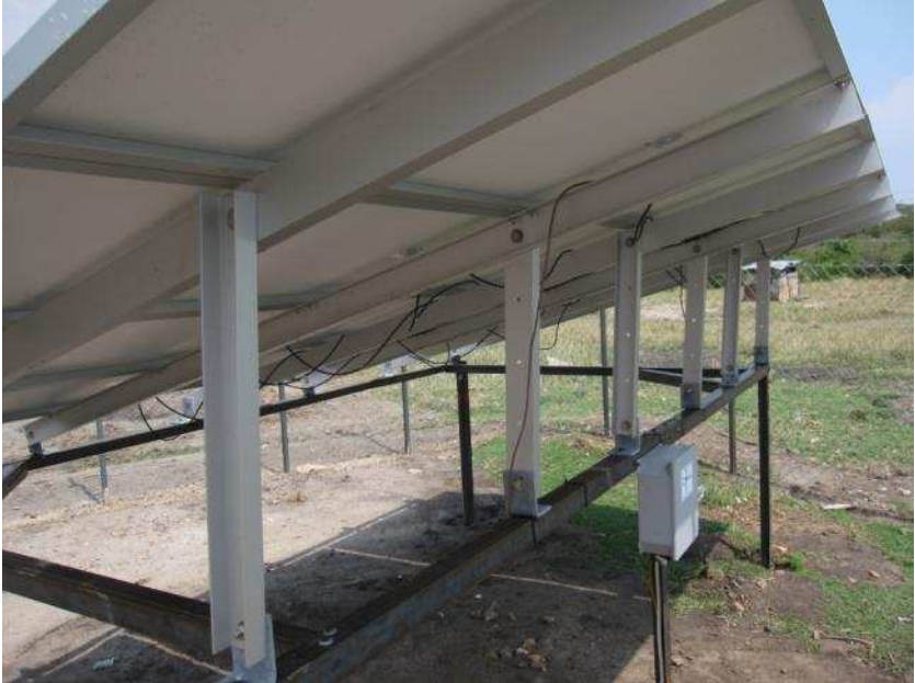
The solar panels from below. The panel control was bolted to the metal frame.
